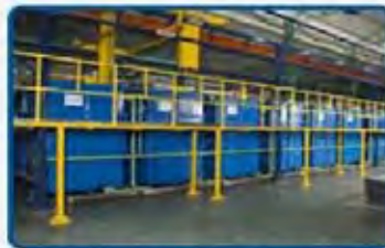
Pre treatment system with PLC based transporter
